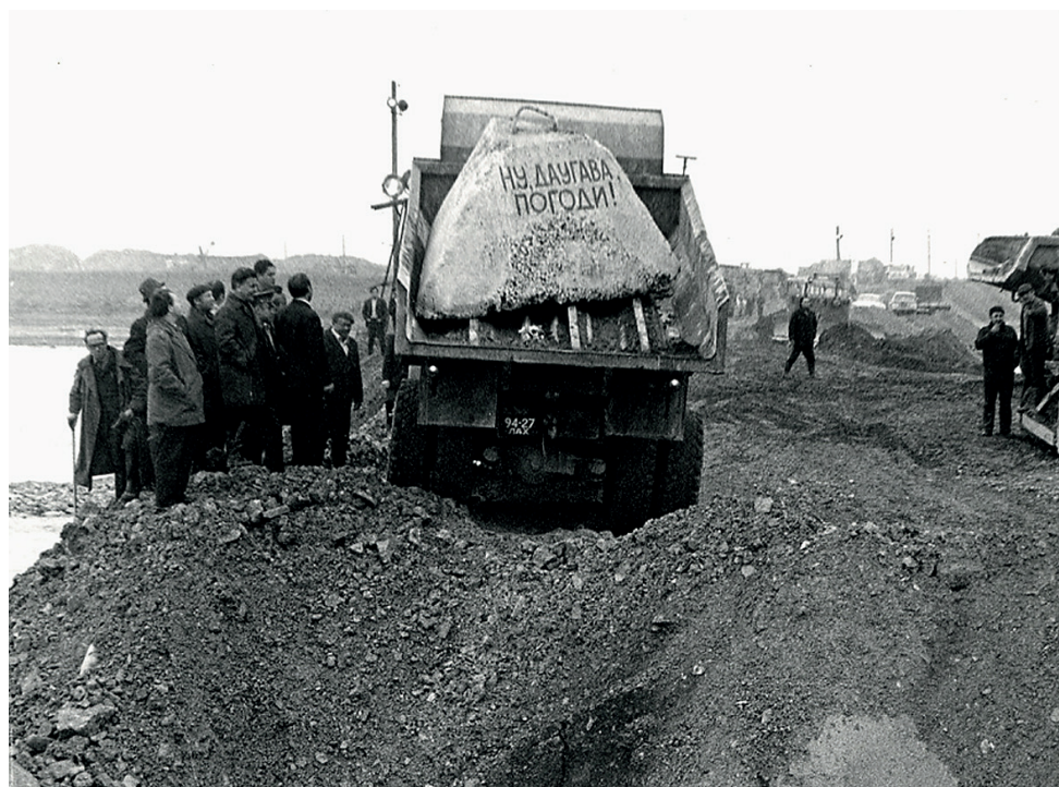
Figure 6. Photo from Riga HPP building in 1974. Inscription on stone in Russian “Well, the Daugava, wait!”. Available: http://www.latvenergo.lv/hesture/hes_rigas.html (viewed 07.11.2016.)
